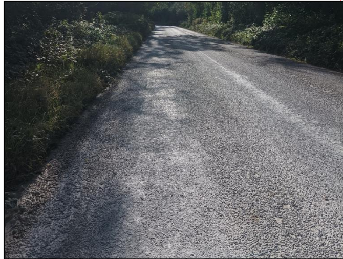
Photograph 14: View South of L1222 Ravelling
