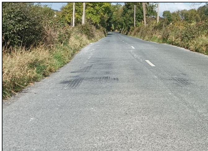
Photograph 5: View North of L1222 Surface Deterioration (Depression)
