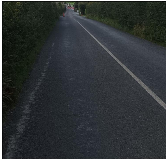
Photograph 27: View South of L1220 Ravelling
