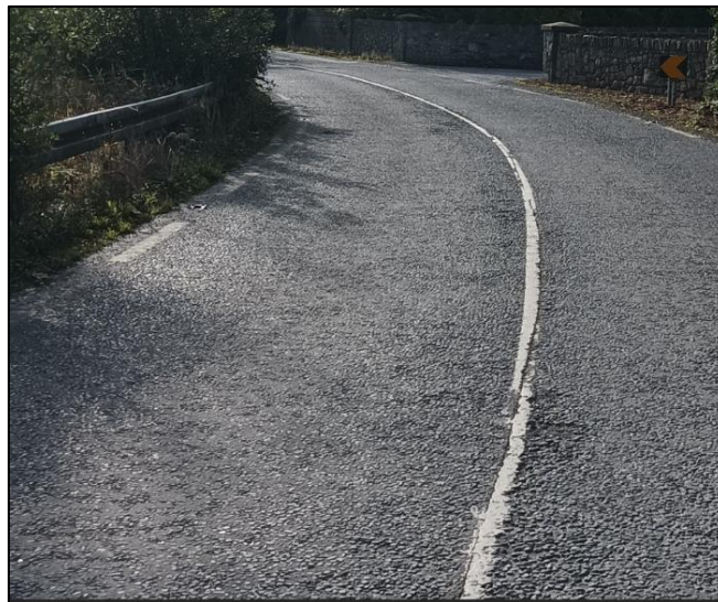
Photograph 1: View South of L1222 Ravelling from Southside of N69 Junction Area
