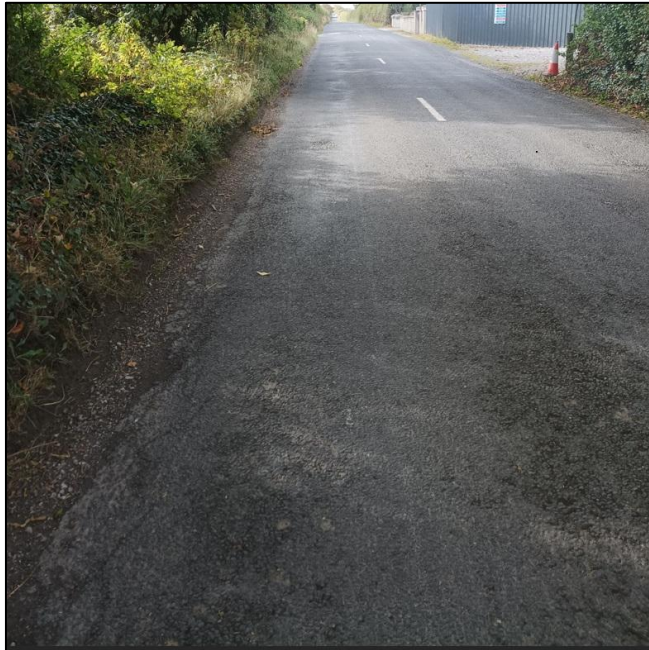
Photograph 24: View South of L1220 Ravelling and Edge Break Up
