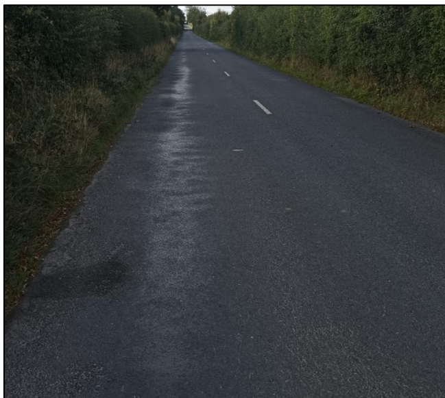
Photograph 25: View South of L1220 Ravelling, Rutting and Edge Break Up
