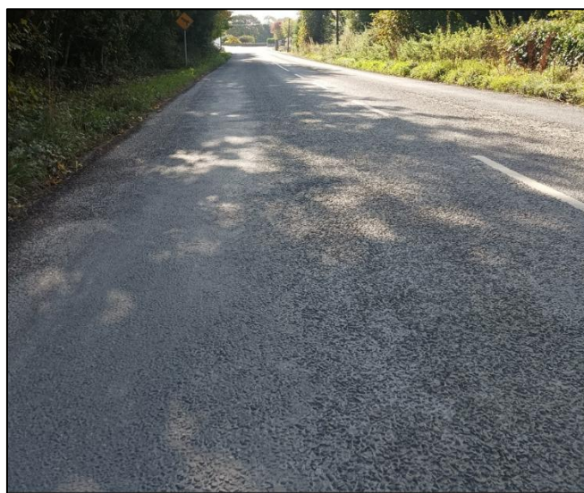
Photograph 18: View South Within Creeves Cross 50 km/hour Zone of L1222 Ravelling
