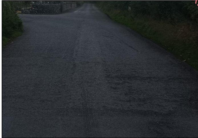
Photograph 30: View East of L1219 Ravelling and Patching
