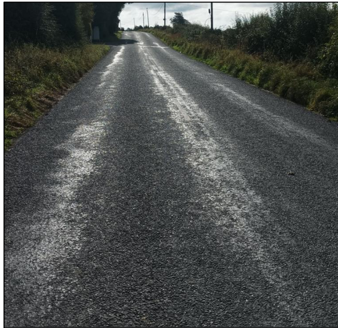
Photograph 4: View South of L1222 Ravelling
