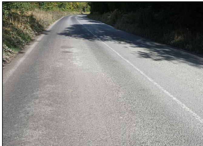
Photograph 15: View South of L1222 Ravelling
