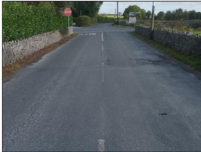
Photograph 20: View North Within Creeves Cross 50 km/hour Zone of L1220 Ravelling and Patching
