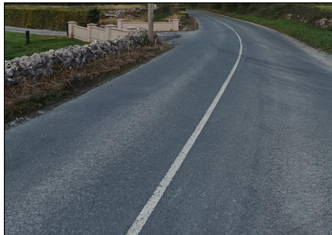
Photograph 7: View North of L1222 Ravelling
