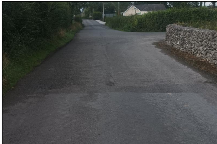
Photograph 31: View West of L1219 Ravelling and Patching
