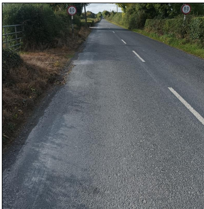
Photograph 23: View South Within Creeves Cross 50 km/hour Zone of L1220 Ravelling and Edge Breakup
