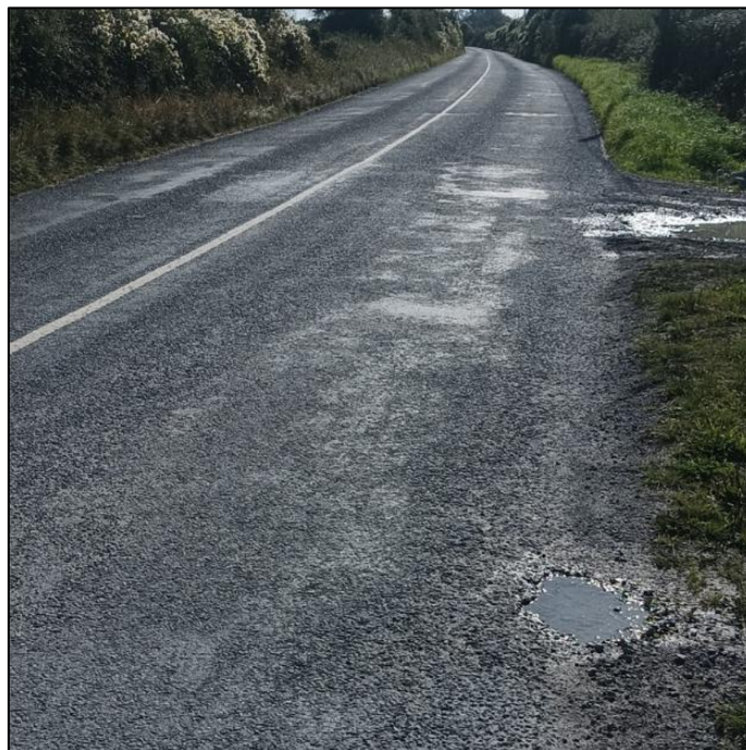
Photograph 9: View South of Potholes on West Edge of L1222
