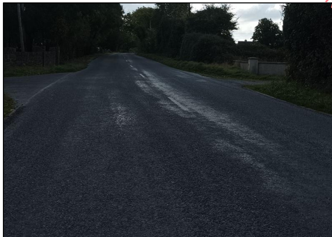
Photograph 10: View South of L1222 Ravelling
