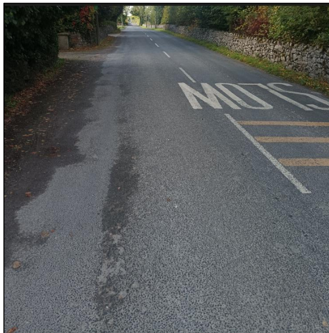
Photograph 21: View South Within Creeves Cross 50 km/hour Zone of L1220 Ravelling
