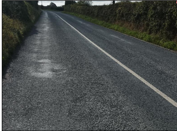
Photograph 8: View South of L1222 Rutting and Ravelling
