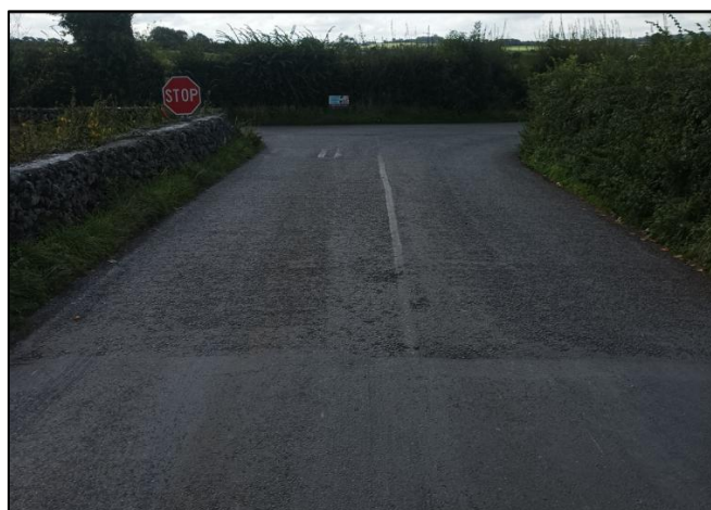
Photograph 29: View South to L1219 Junction of L1220 Patching and Ravelling
