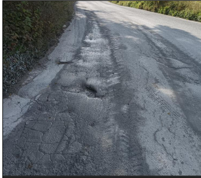
Photograph 12: View South of L1222 Potholes and Cracking on South Side of Roadstone Joseph Hogans Quarry
