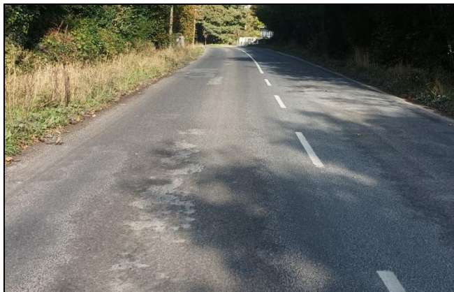
Photograph 17: View North Within Creeves Cross 50 km/hour Zone of L1222 Ravelling
